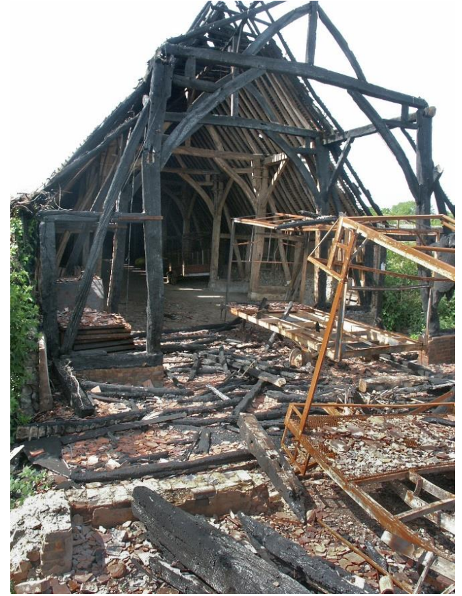
Pl 5: North end of barn after the fire of 2003.
