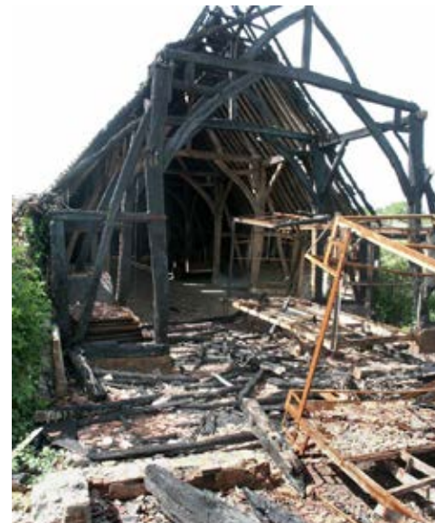
Figure 24 | North end of the barn post fire
